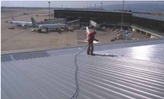
Roof waterproofing of Terminal 2, Barcelona airport, with Impermax Plus System from Krypton Chemicals
