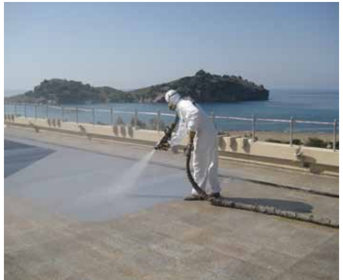
Polyurea Quick Spray is applied to concrete, metal or foam by high pressure spray units
