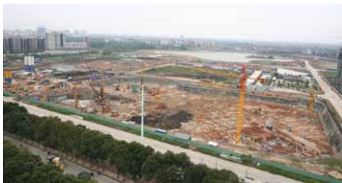
BAUER Vietnam Ltd. carries out foundation works for luxury apartment towers in Hanoi
