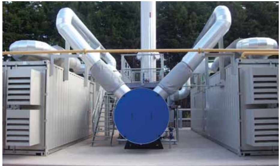
Edina UK received the second order for power generation from sewage gas
