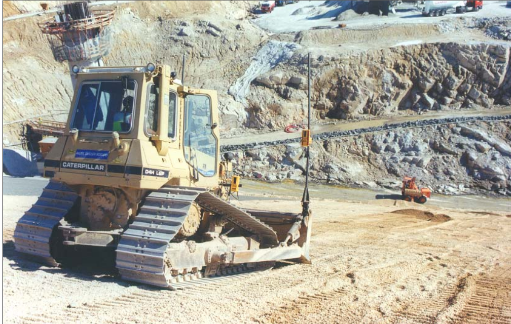
La Galaube Dam- Upstream face - July 2000 Laying 0/20 crushed limestone with leveling by laser
