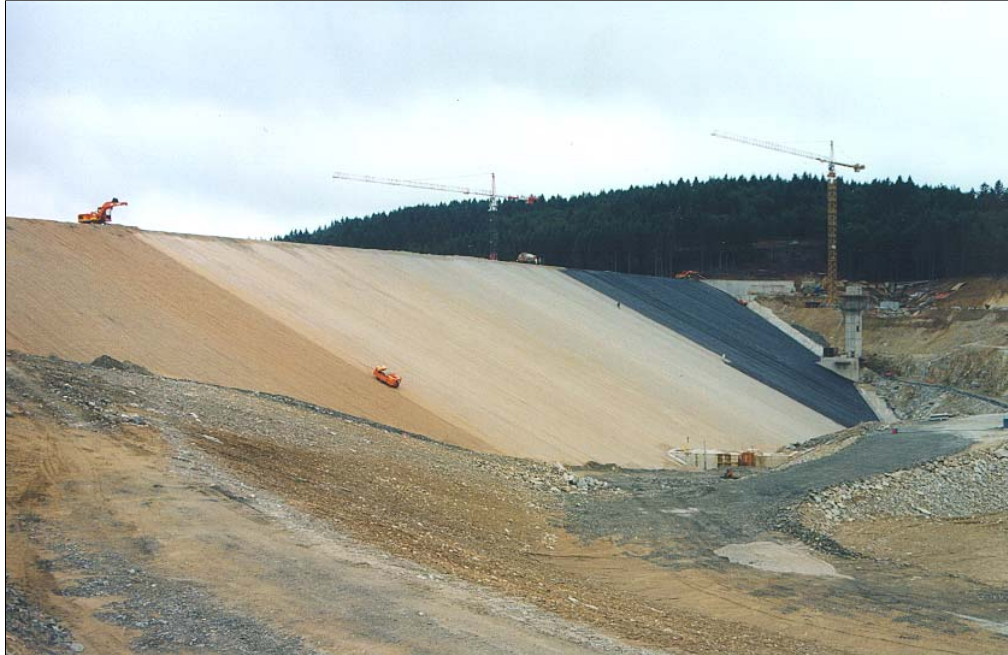
La Galaube Dam- Upstream face - July 2000 Compaction of 0/20 and impregnation with bitumen emulsion
