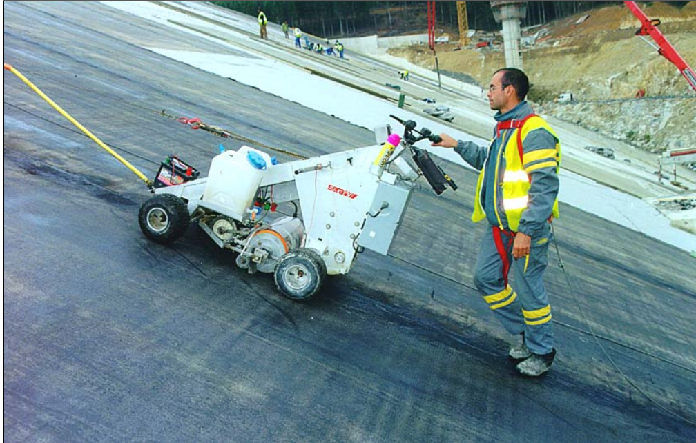
La Galaube Dam - October 2000 COLETANCHE NTP3 – Automatic control of seams by CAC 94
