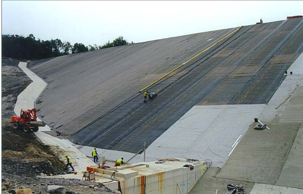
La Galaube dam - October 2000 COLETANCHE NTP3 - Control automatic of joints by CAC 94
