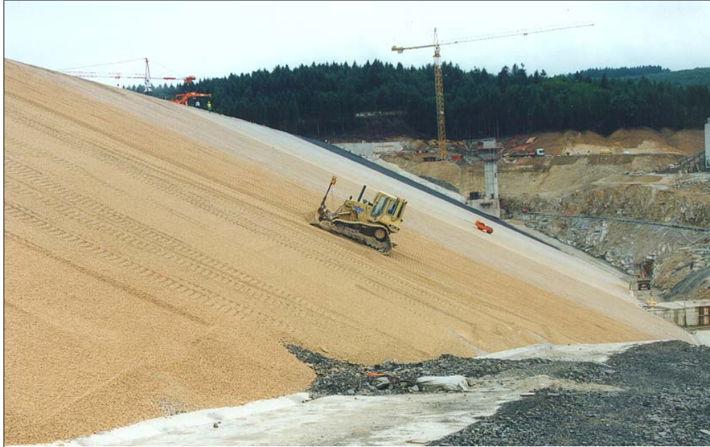
La Galaube Dam- Upstream face - July 2000 Laying 0/20 crushed with leveling by laser apparatus
