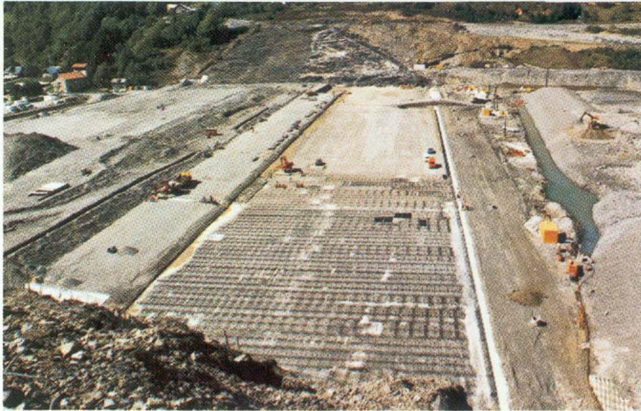
Protection of the foundation of the supporting mass of the Vernet dam, E.D.F. development, Grand-Maison site (France).
