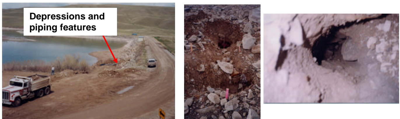
Figure 1. Surface Depressions and Vertical Piping Features at Nilan East Dam
