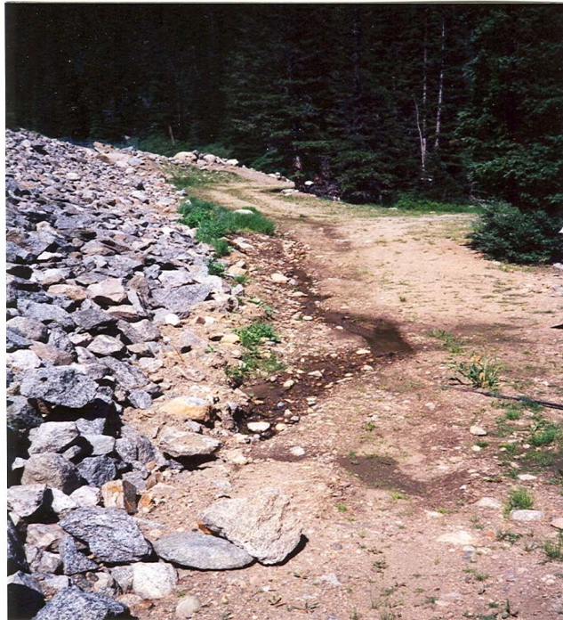
Figure 2. Seep at downstream toe of dam prior to rehabilitation
