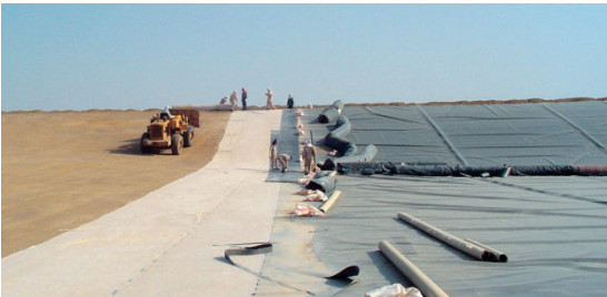
Saudia Arabia Installation of Carbofol® over Bentofix® GCL in a gold mine
