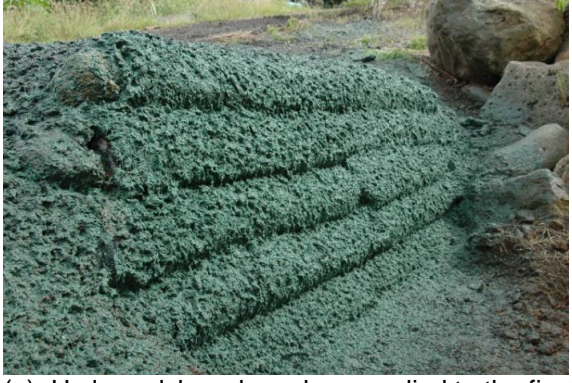
(e) Hydromulch and seed are applied to the final sock-module MSE wall.
