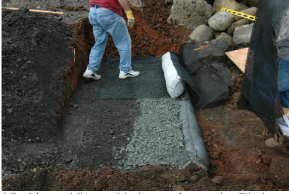
(d) After adding a thin layer of granular fill, the next row of modules is placed, and so on.
