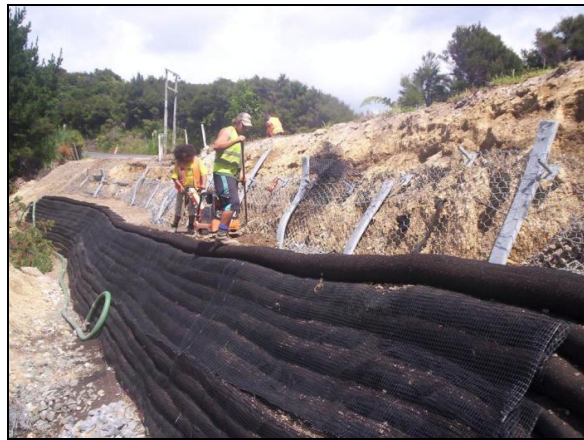
(a) Due to inadequate space for a wide enough reinforced backfill zone, short geogrid wraps are attached to a slope-anchoring system based on soil nails installed in the backslope.
