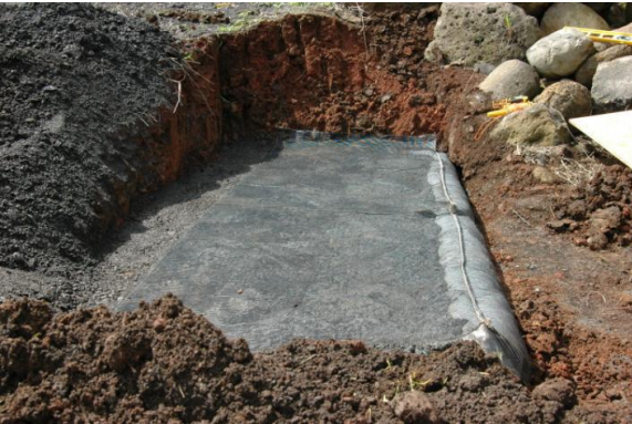
(c) Upper geogrid extension of module is laid back over the backfill and smoothed.
