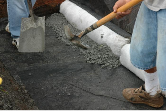
(a) Granular fill applied on top of the lower geogrid extension of first module row.
