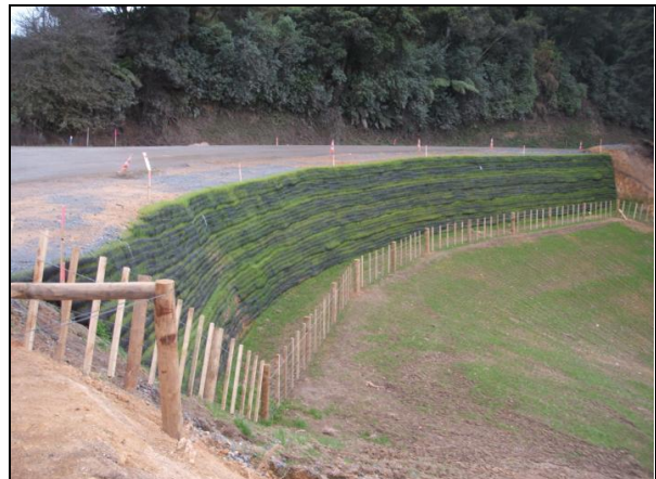
(b) Completed MSE structure with new vegetation growth on the compost-sock facing.
