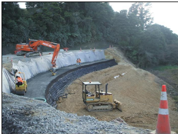
(a) Compost socks at the face are wrapped with geogrids incorporated into a compacted, reinforced zone of granular backfill.
