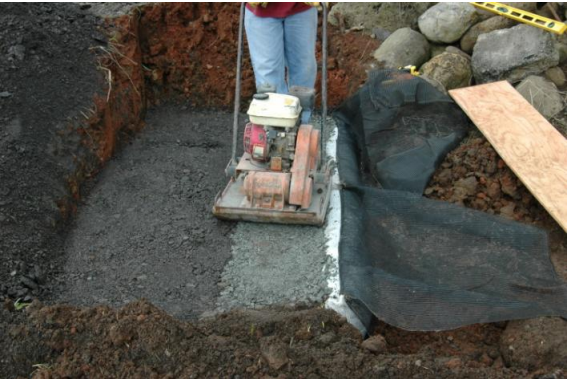
(b) Compaction of layer/lift of granular backfill behind module (no bracing form needed).
