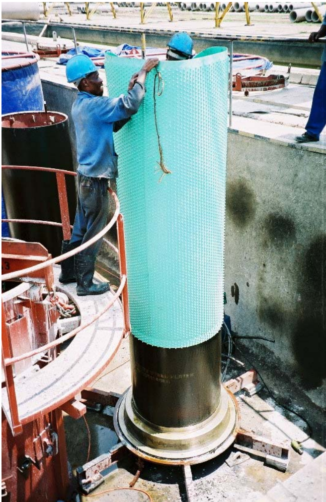
Engineered Linings' AKS CPL being fitted to the mandrel which forms the I.D. former for the concrete sewer pipe. Note the tight fit and the anchor knobs referred to in the text
