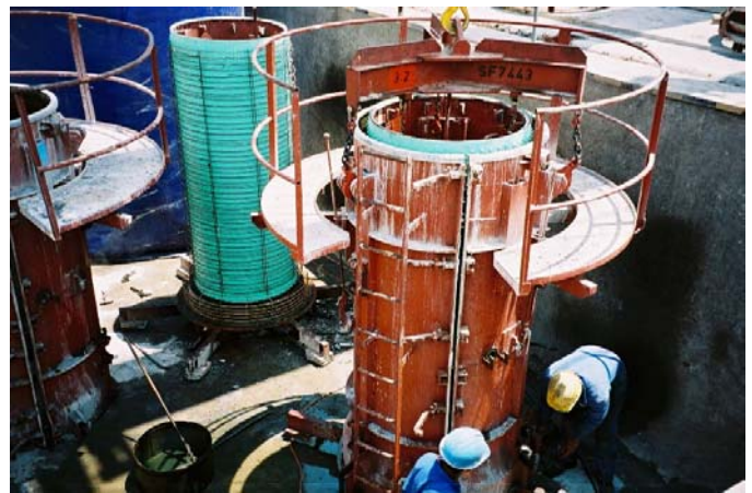
A view of the AKS mould, shuttering, HDPE liner and reinforcing, all being combined to produce the resultant CPL system.
