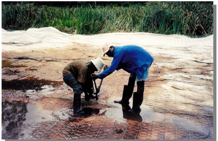
Fixing panels of Flexmesh over the wetland. Note wire mesh and transverse steel rods over the geotextile.
