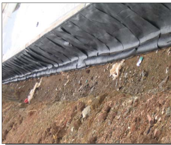
outside of canal wall The project comprises 120,000m 2 HDPE and 45,000m 2 Hidrain 500.
