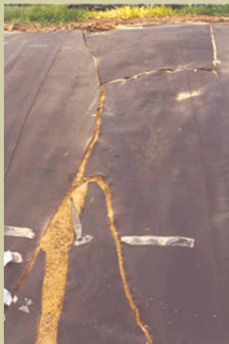
Photo 4, PP failure in USA, circa 1993.
