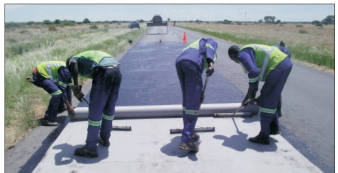
Fibertex geotextile stress relieving and waterproofing layer placed onto the road surface, Route B1 Namibia - 2012
