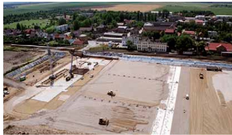
Sinkhole protection at railway junction
