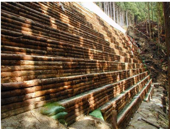
Retaining wall with a near-vertical wall face constructed with recycled plastic logs.
