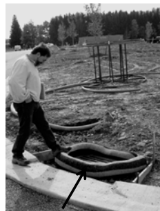
This fiber log has NOT been applied properly!
