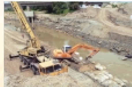
Installation of Secutex® Sand containers as down stream dam to capture sediments
